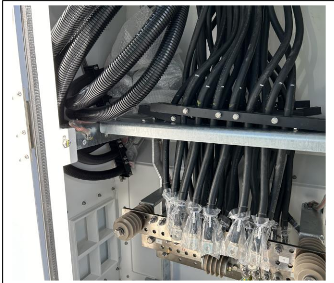
2784 - Wiring from Arm to Pedestal Base on Buss Bar Side
