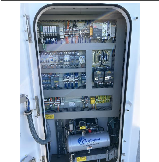
2749 – Electronics Side of Pedestal Base
