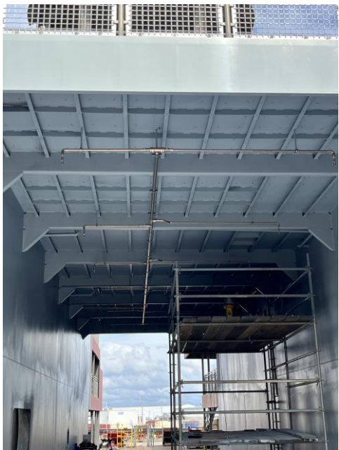
5133 – Fire Suppression piping down vehicle alleyway
