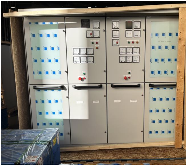
5233 – Part of PEMS Switchboard
