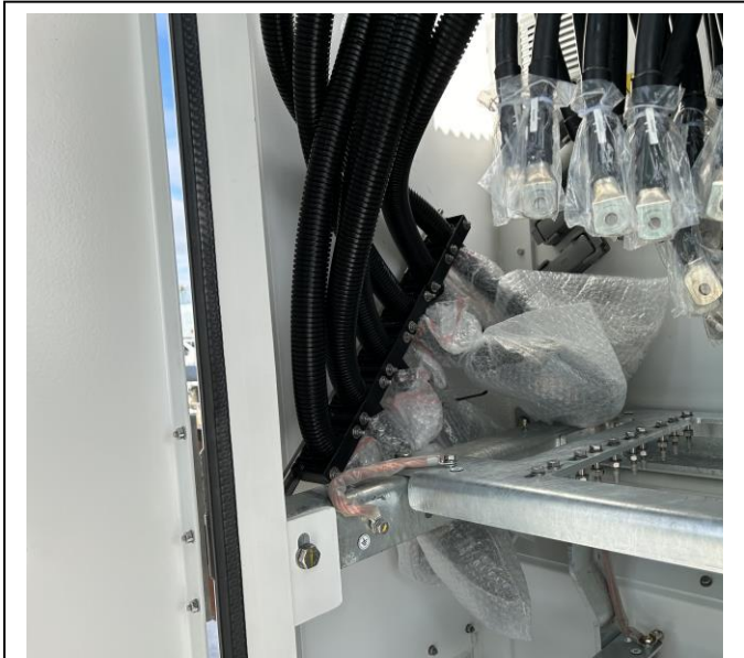
2776 - Wiring from Arm to Pedestal Base on Buss Bar Side
