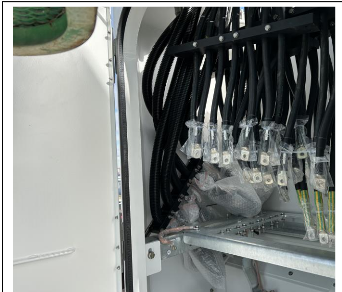
2777 - Wiring from Arm to Pedestal Base on Buss Bar Side
