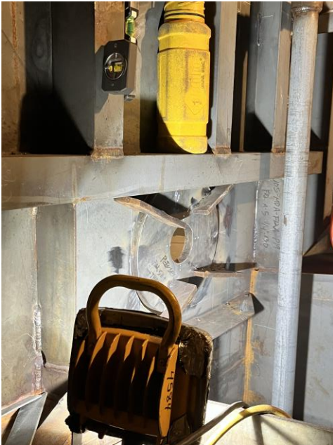
5173 – Rudder Post Area in Lazarette
