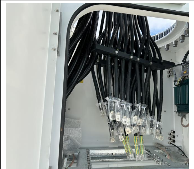
2775 – Wiring from Arm to Pedestal Base on Buss Bar Side
