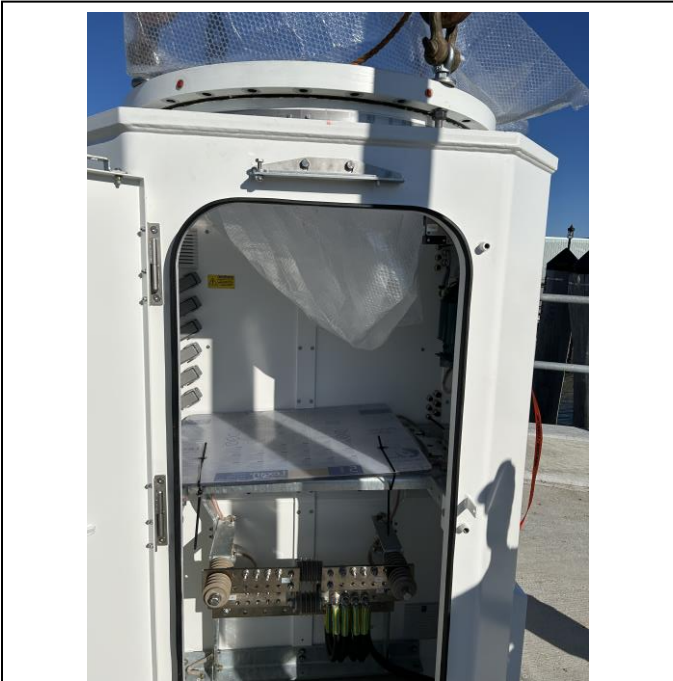
2747 – Buss Bar Side of Pedestal Base
