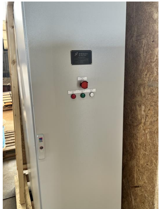
5234 – Propulsion Motor Cabinet
