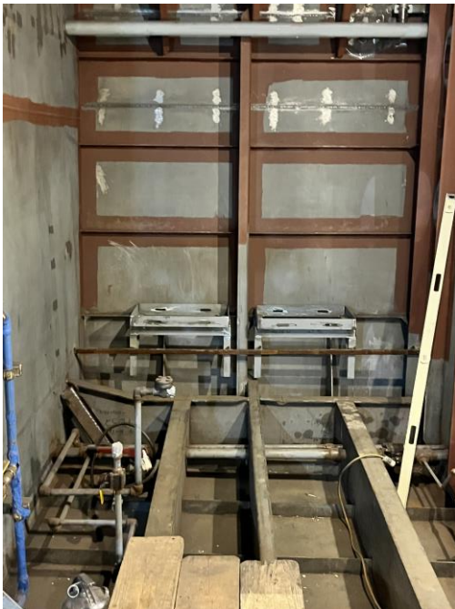
5297 – Generator Bay in the Engine Room
